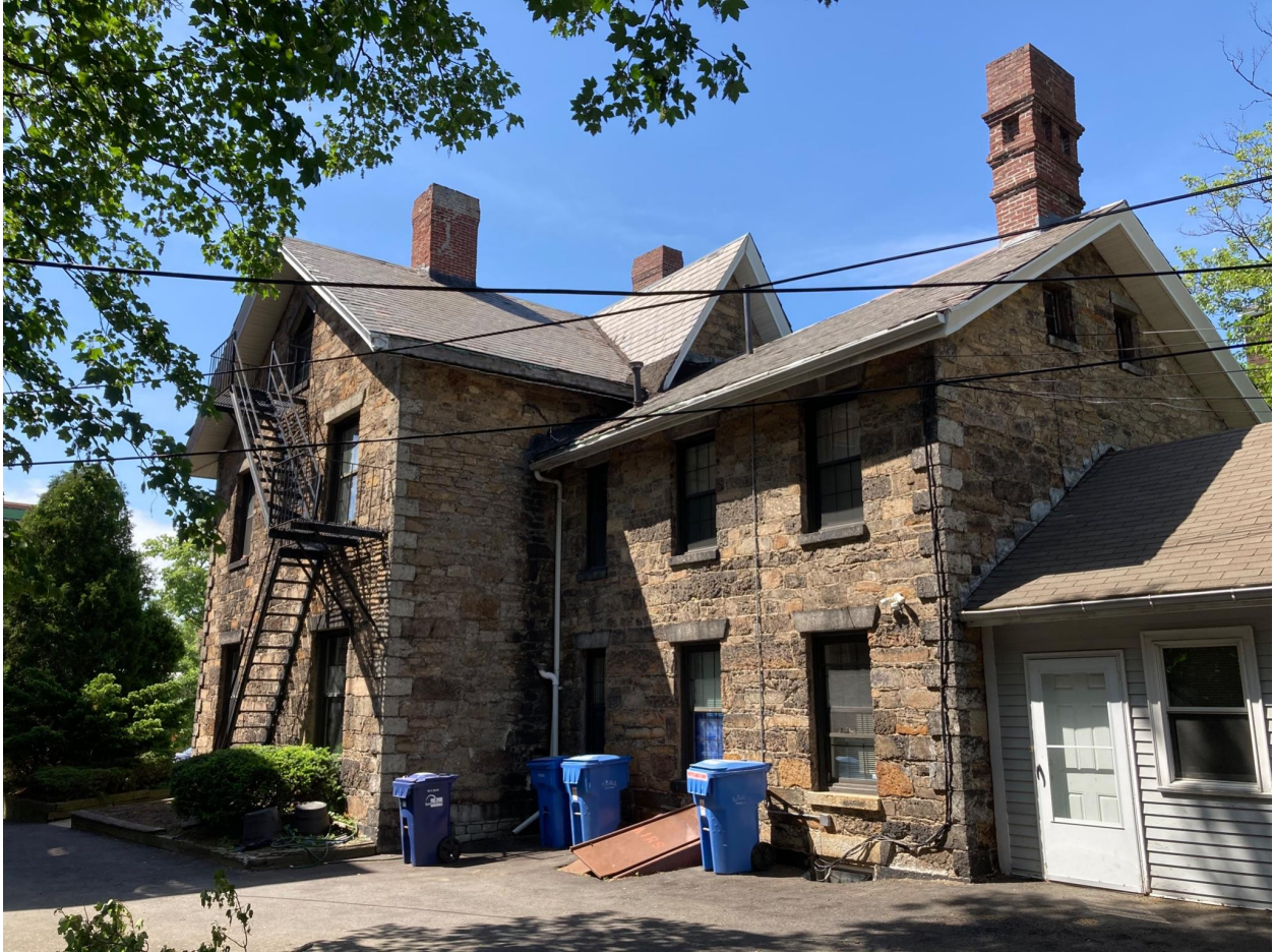
Figure 9: South and east elevations of main block and rear wing; partial south elevation of one-story addition
